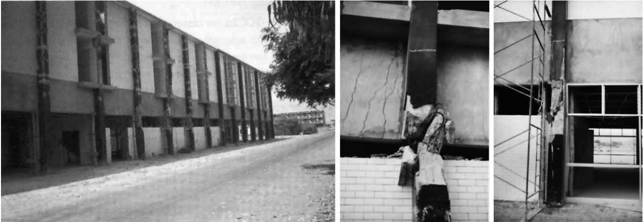
Figure 1: The two extreme columns are long and have not failed. The central columns, trapped by the white wall, are short and their lateral inflexibility is about 40 times greater than the inflexibility of the long columns. They attracted a major percentage of the seismic cut and failed (Photos: Julio Kuroiwa, Disaster Reduction Book - Living in Harmony with Nature , p. 172)
