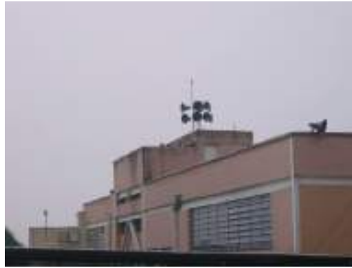
Photo 4.9: Sirens and rain meter in the remote alarm unit in the Morro da Formiga community. The equipment was installed on the terrace of a local school, also used as a temporary refuge in the event of extreme weather.
